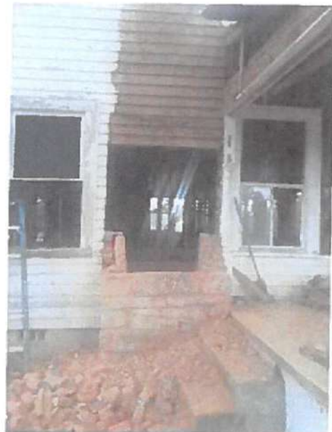
This photo shows the lower section of one chimney. All three chimneys have a granite base and firebox inside.
